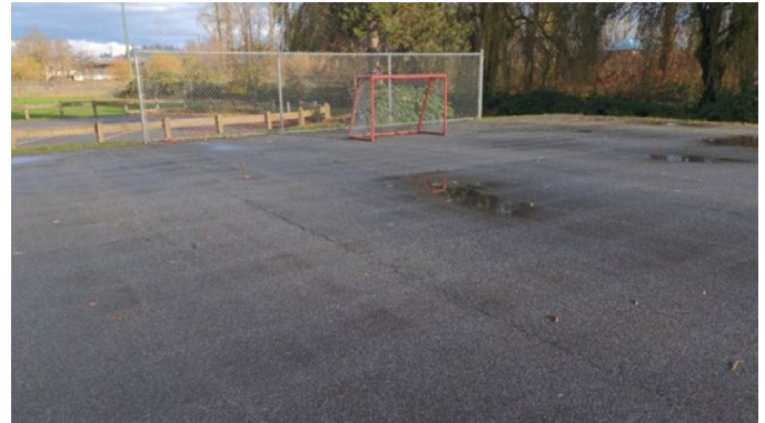
Matsqui Village Park: Example of cracking paved surface and water pooling
