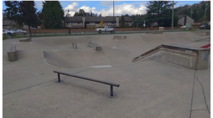
McMillan Park: Example of skatepark with some minor surface cracks
